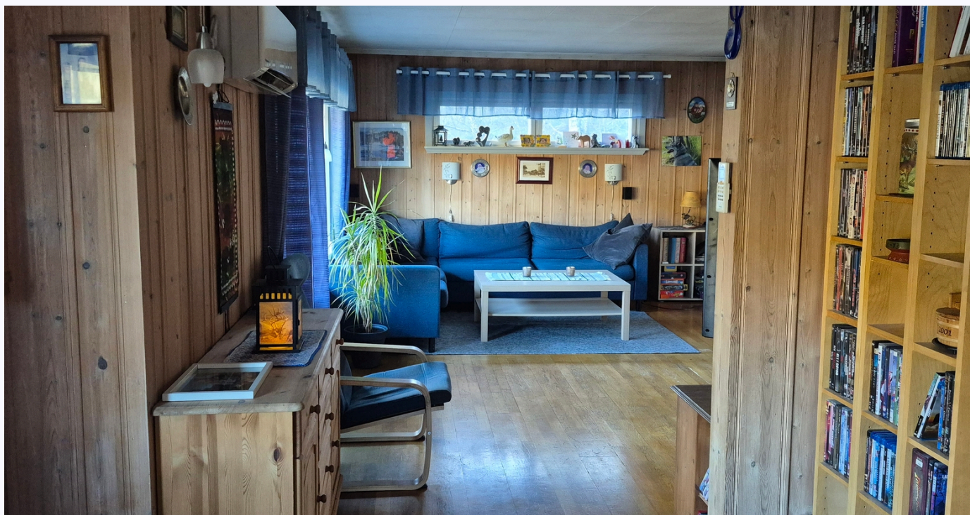
Stue - m Pannasonic varmepumpe (2017)
